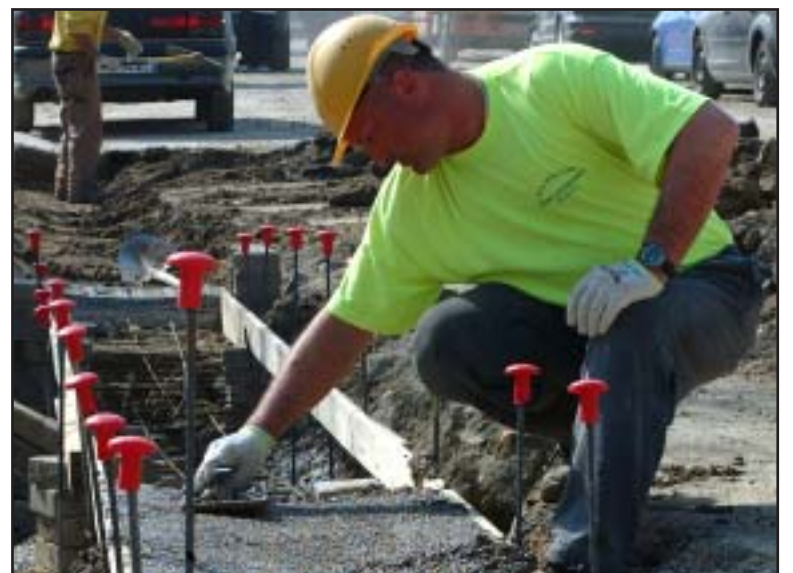
Luca Bergamo, a contractor with Bilfinger-Berger, smooths out the concrete drainage portion of the roadway along Raffaello Sanzio in Villaggio. Residents along that street will soon have the road blocked off so the road can be repaved.
